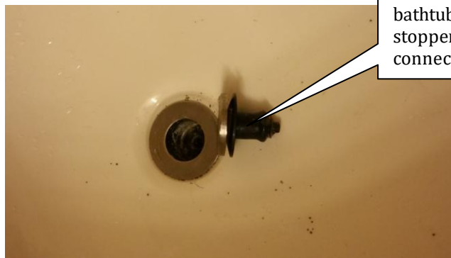
1st floor shower faucet not mounted correctly.
