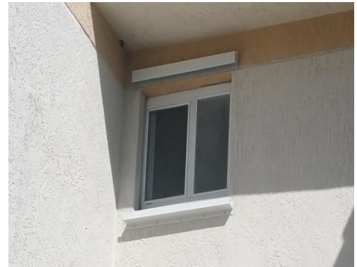
Hurricane shutter mounts
