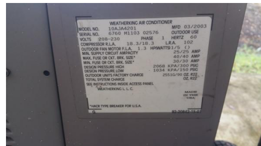
Compressor unit label 2003
