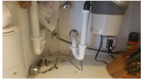
Copper & PVC plumbing
