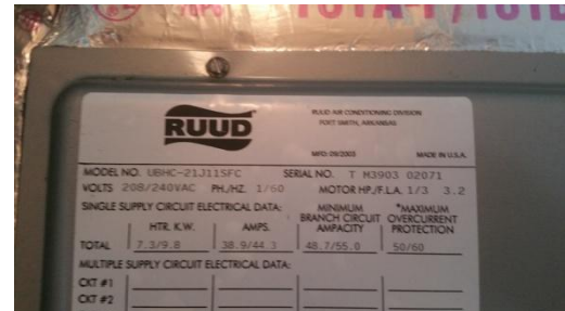
Air handler label 2003
