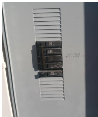
GE Main circuit panel
