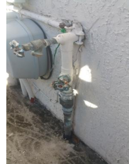
Copper water main
