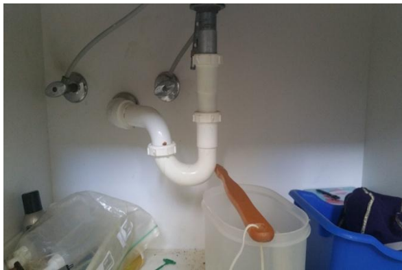
Copper & PVC plumbing
