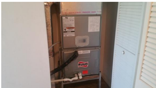
Air handler unit
