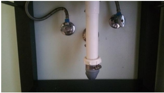
Copper & PVC plumbing
